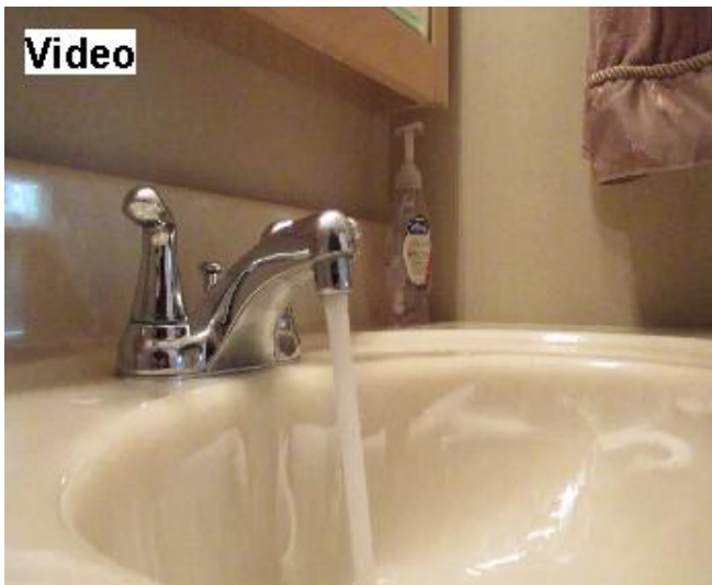
Bathroom #1 no pressure loss when toilet is flushed
