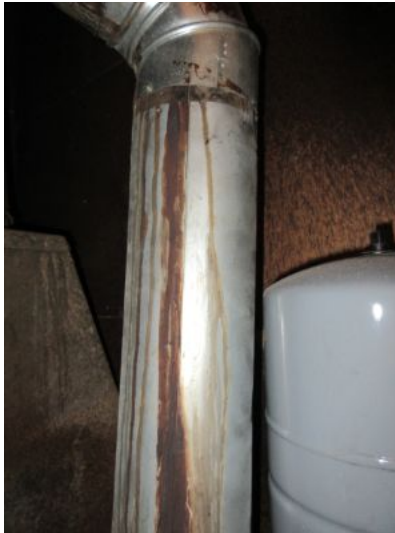
Boiler Flue Pipe
