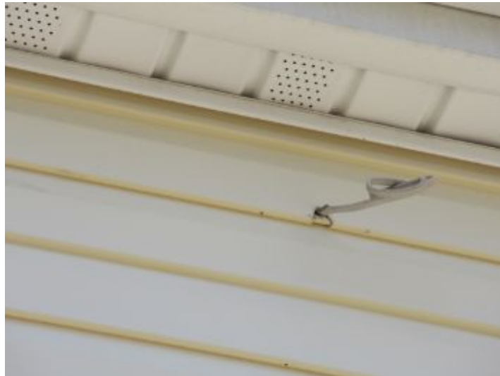
Missing light fixture
