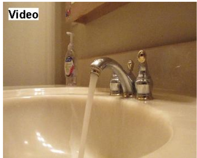
Bathroom #2 No pressure loss when toilet is flushed
