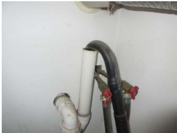
Laundry Washer Connections & Drain
