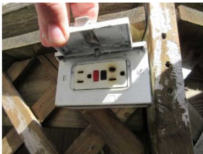
Damaged pool side GFCI
