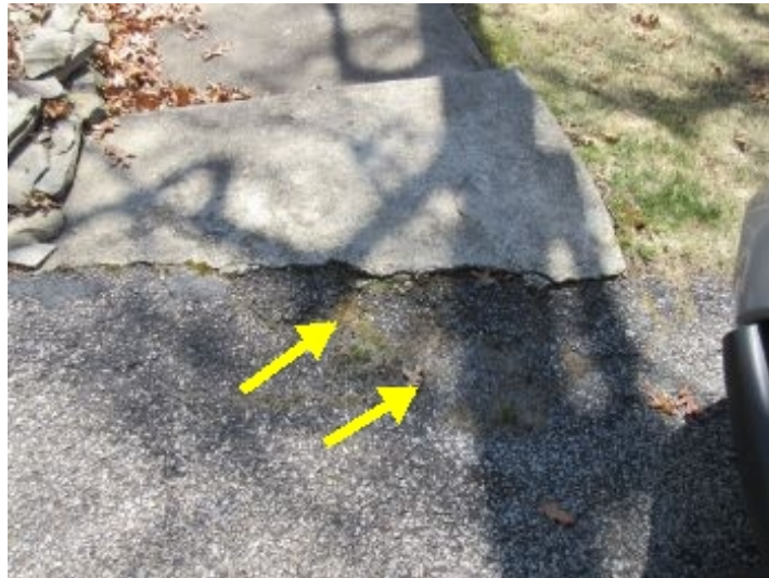
Uneven walking surface
