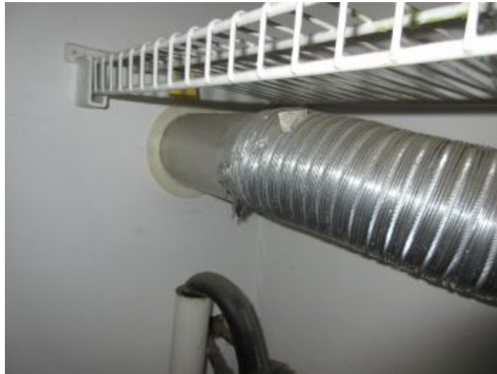
Laundry Dryer Vent
